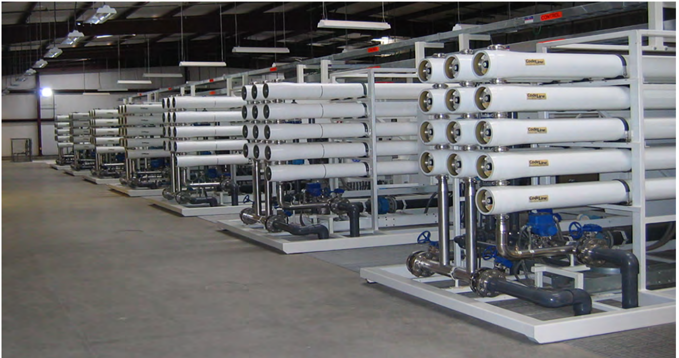
Reverse Osmosis Facility for Direct Potable Water Treatment.
